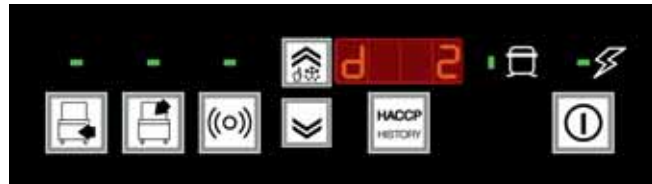
Refrigerated unit control panel
